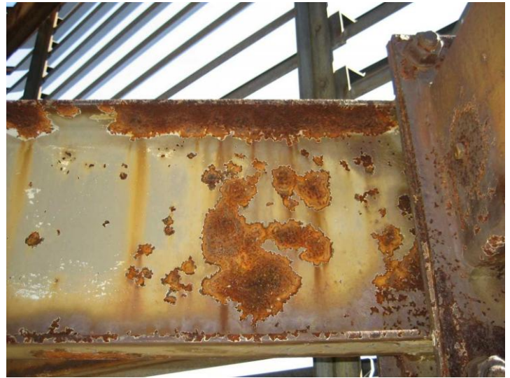
Fig.4. Sample image of steel construction with corrosion
